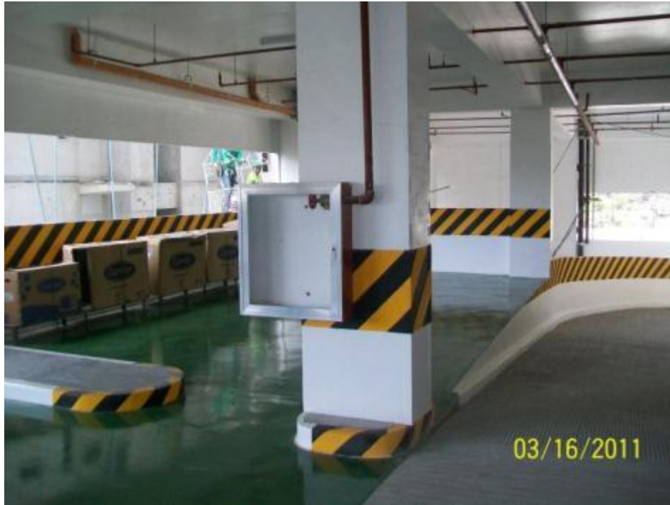
*Fire hose cabinets
