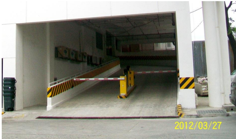
*Installed boom gate
