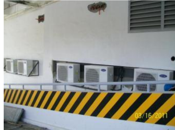
*ACCU units and Generator room
